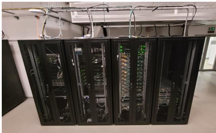
Figure 2: ORO Network infrastructure deployment
